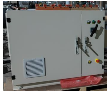
250kW Semi sealed/fully sealed 半密封/全密封
